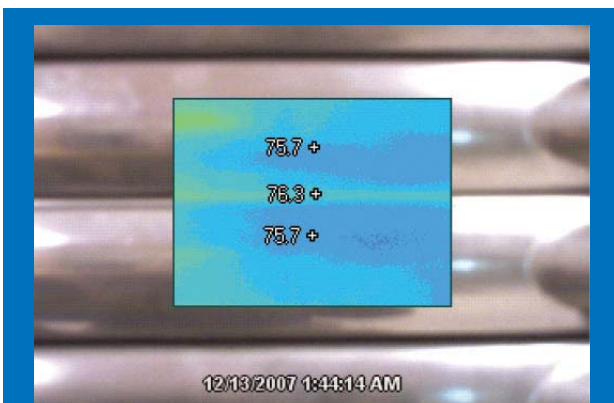
In a data centre with a conditioned airflow temperature of 72°F (22°C), a series of HotLok Blanking Panels are installed. The consistent temperatures shown on the face and gaps between the panels reveal the highly effective sealing technology.
