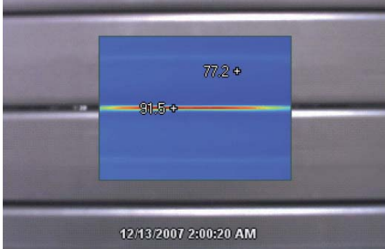
In a data centre with a conditioned airflow temperature of 72°F (22°C), and a series of non-HotLok Blanking Panels installed, the measured temperature of the heat radiating through the horizontal gaps is 91.5°F (33°C), which is much higher than the ASHRAE - recommended 77°F (25°C).
